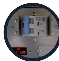
Breaker of batteries
